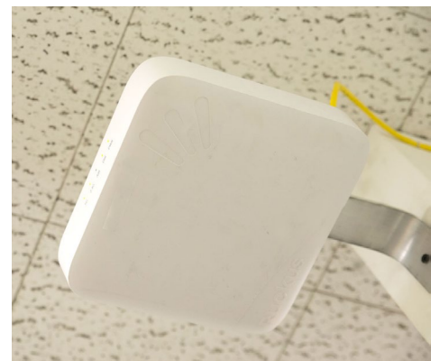
BELOW: 802.11n and 802.11ac APs are mounted dome-down with standard 802.3af PoE connections.
